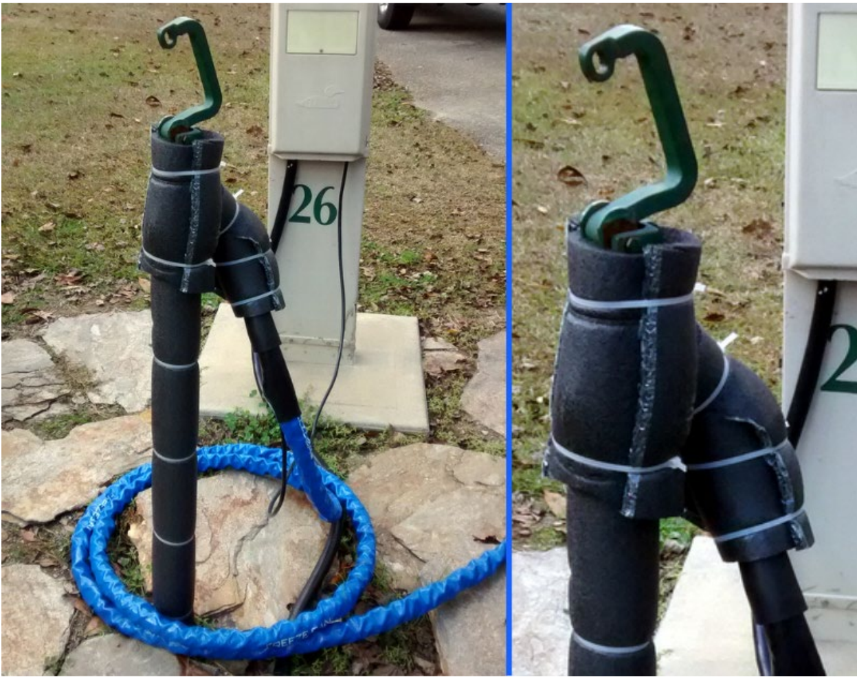
Insulate the water hydrant pipe and hydrant head with ½ in foam or some other insulation material
